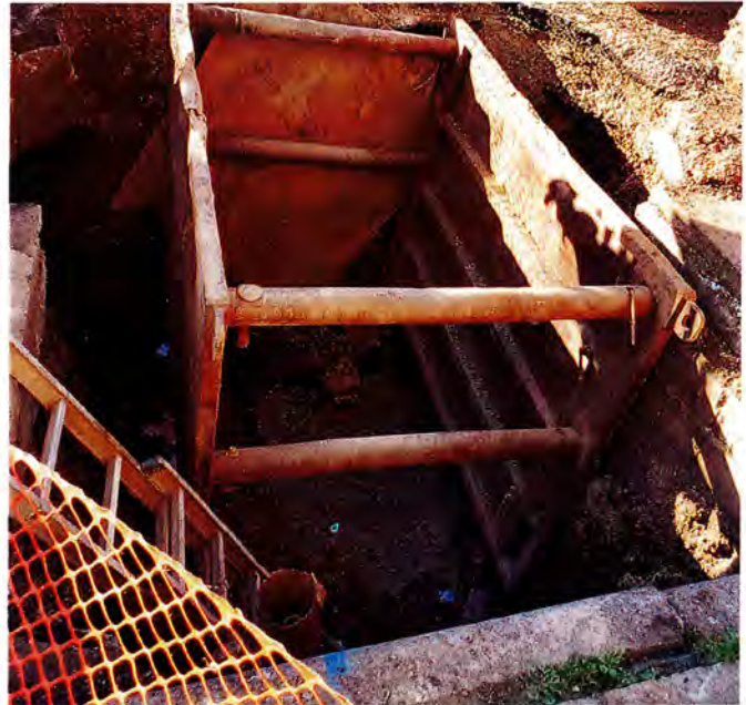
Existing watermain below south lanes.
