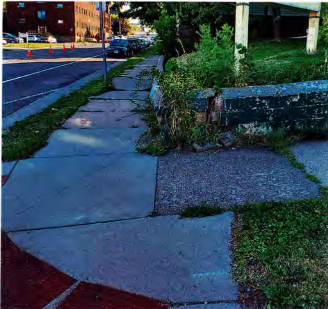
Failed retaining wall at Eighth Avenue E.
