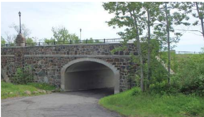
Poor approach sight lines for vehicular and pedestrian traffic at 10th Street bridge underpass
