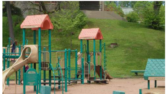
Existing playground does not meet ADA accessibility requirements
