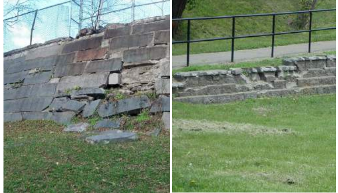
Retaining wall Infrastructure in need of tuck pointing repair or replacement
