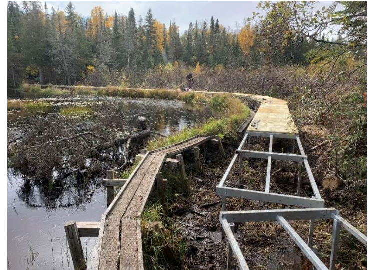
Before & after of old Boardwalk being replaced with longer lasting and safer material.
