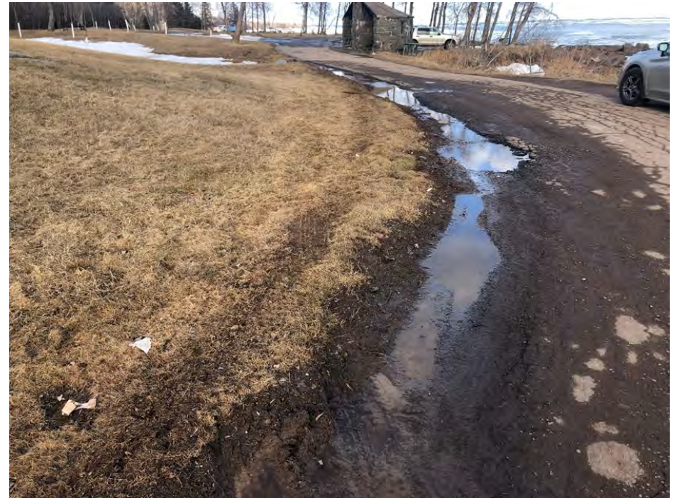
>>Photo Credit: Road erosion, Park Staff
