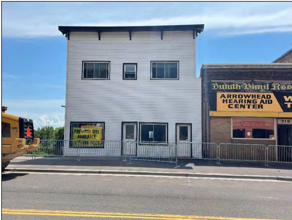
Photograph 18: View of a building in the historic district that is inappropriately wrapped with modern siding, concealing its architectural features preventing the building from conveying its history and architectural style.
