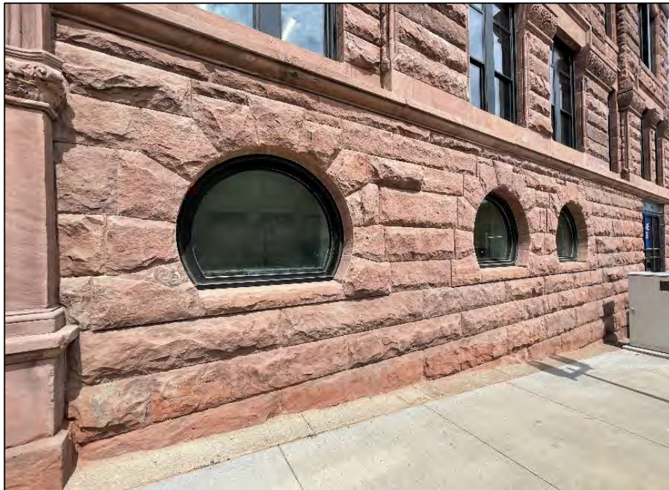
Photograph 13: Decorative rusticated stone elements as seen here, should be maintained.
