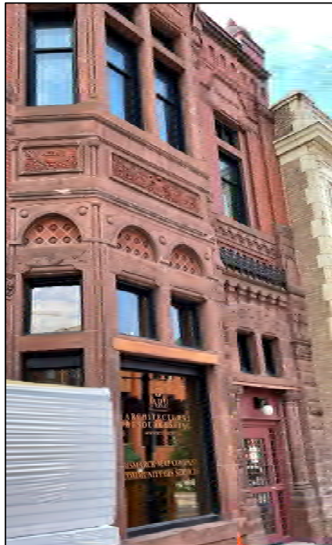
Photograph 17: View of the former Duluth Police Headquarters showing a variety of decorative architectural features including cast iron railing, molded brick and brick corbels, and carved stone.
