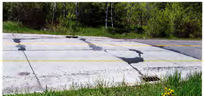
Example of uncontrolled transverse cracking and pavement failure associated with in-place utilities (storm pipe between catch basins).
