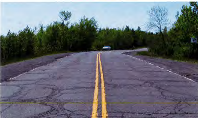
The inplace bituminous pavement near TH 61 is in poor condition with widespread cracking and will be reclaimed as part of the project. Inplace gravel shoulders will be paved.
