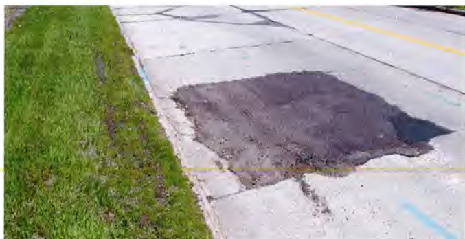
Pavement patching at location of City utility work. There are 12+ such locations along the existing 42-inch water main.
