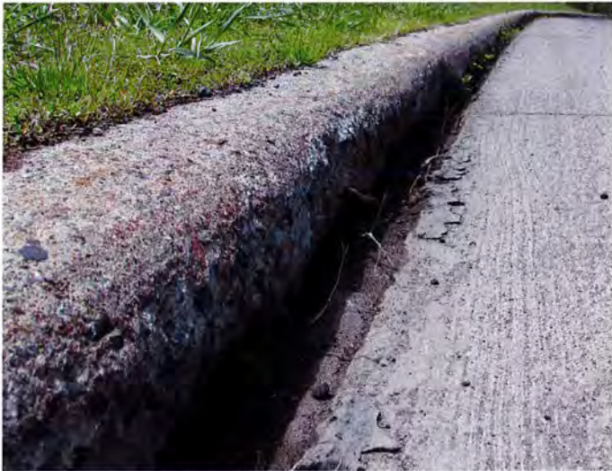
Photo of common curb deterioration with loss of concrete along the curb flow line near the intergral curb joint and exposed tie bars.
