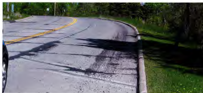
Photo looking east entering the horizontal curve. The pavement and curb in this area is in poor condition as is the similar low lying area further to the east past the roadway high point near the entrance to St. Luke's Clinic.
