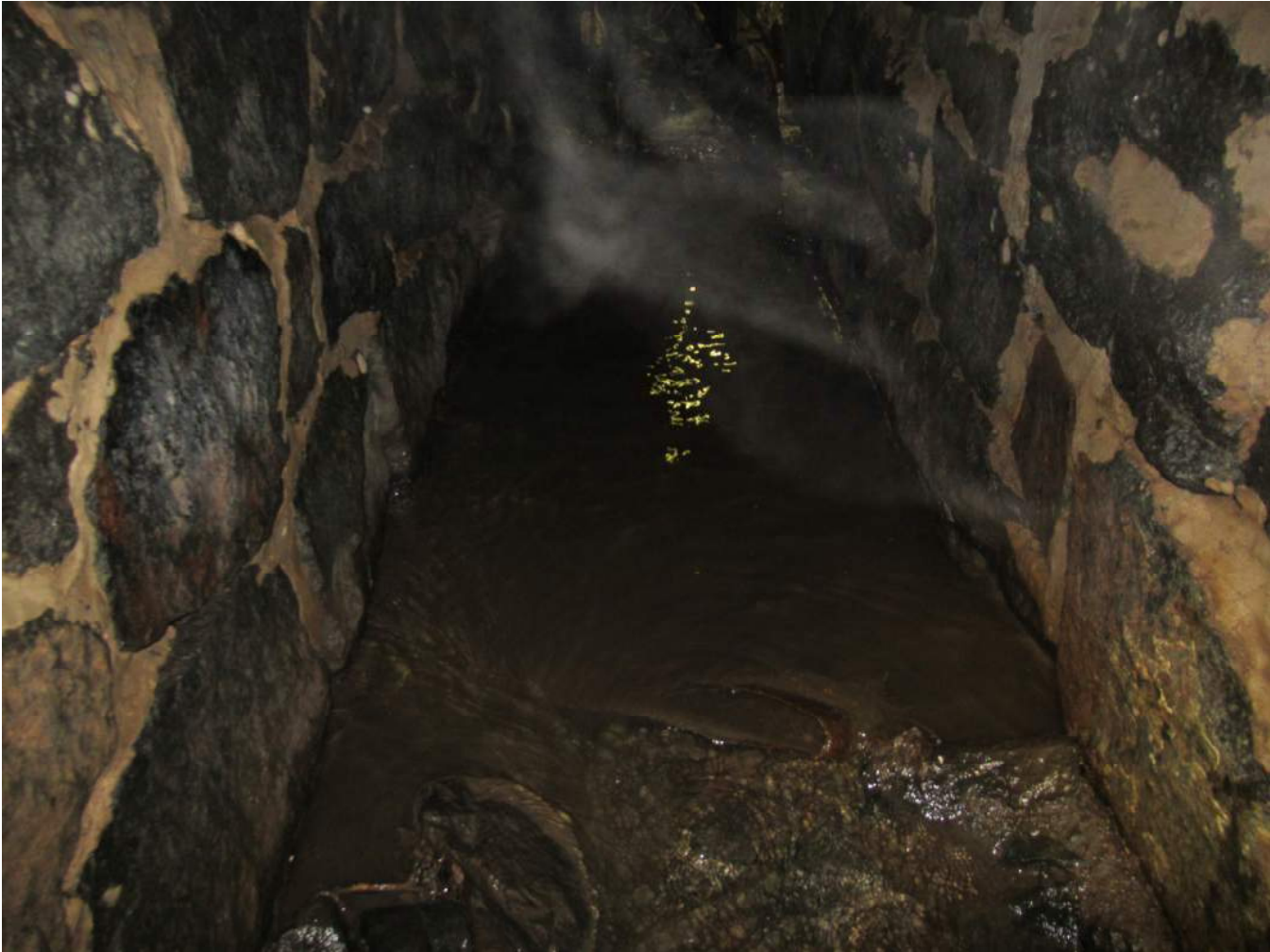
Coffee Creek – Scoured floor
