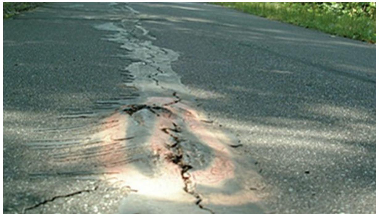
>>Photo Credit: Munger Trail Repair Area; Duluth News Tribune
