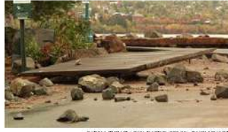
October 2018 Lake Superior storm damage (photo courtesy)
