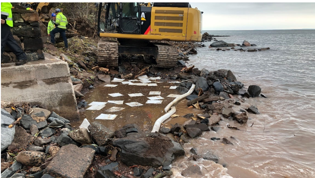
Figure 3: Photo of contamination area and containment efforts, looking East.
