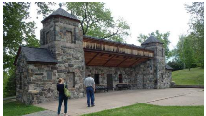
No operational restroom facilities in pavilion building
