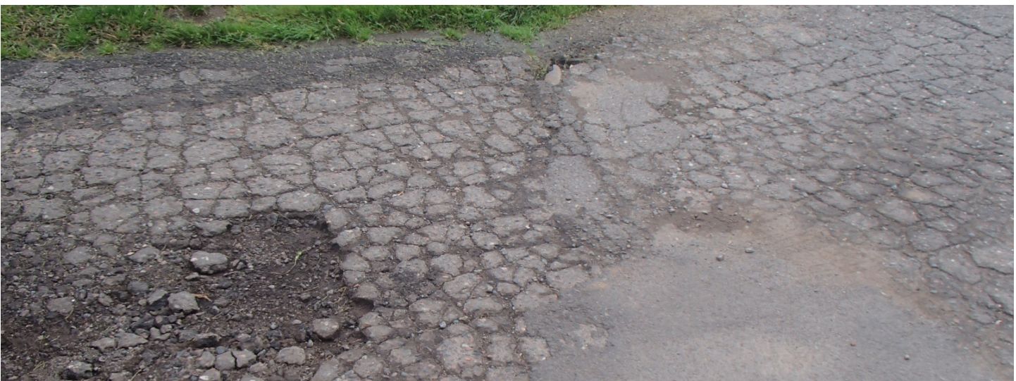
Deteriorated pavement will be replaced to improve ride and surface drainage.
