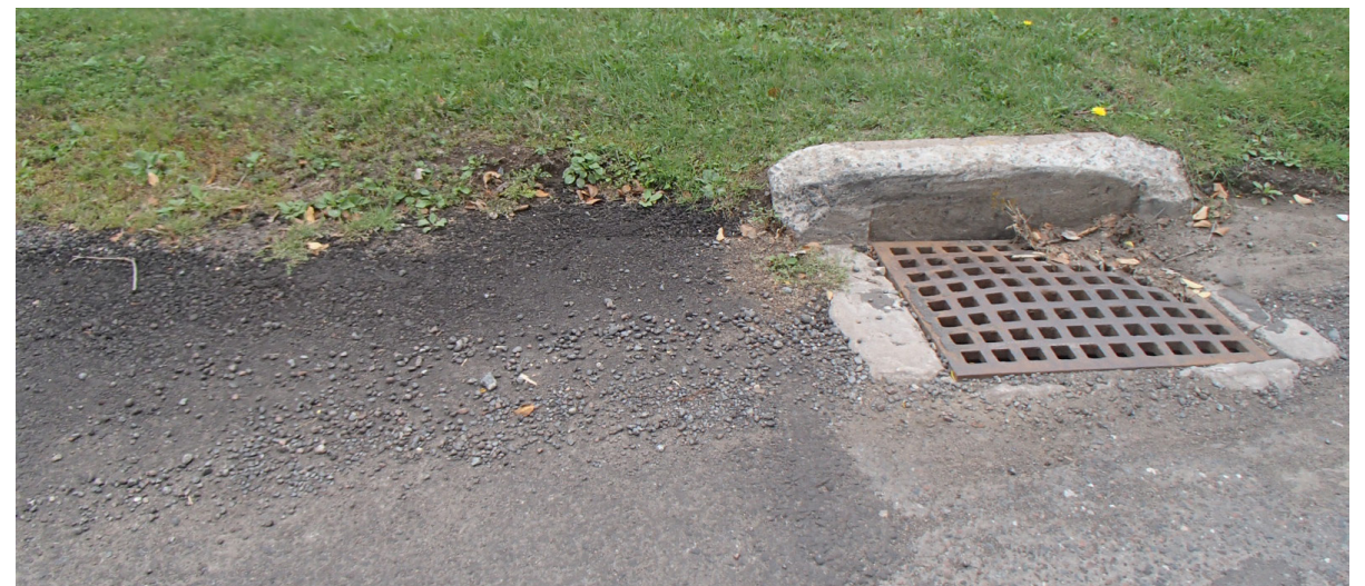
New curbs and storm sewer structures will improve surface drainage and pavement quality.
