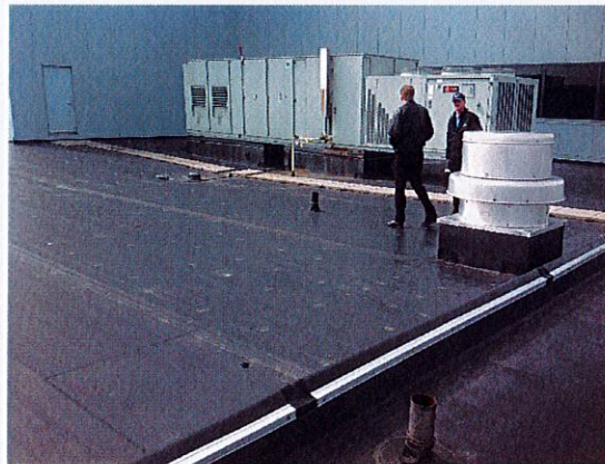
Observation #2 Siding should be installed on these walls to eliminate leaking
