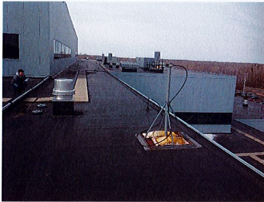
Observation #1 Most of the field seams have been overlaid. There are still quite a few curbs and edge flashing to address
