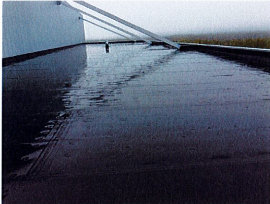
Observation #1 All the field seams have been stripped in on this section
