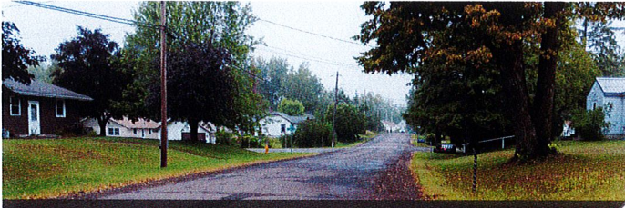
Eklund's pavement is in poor condition with shallow stormwater ditches.
