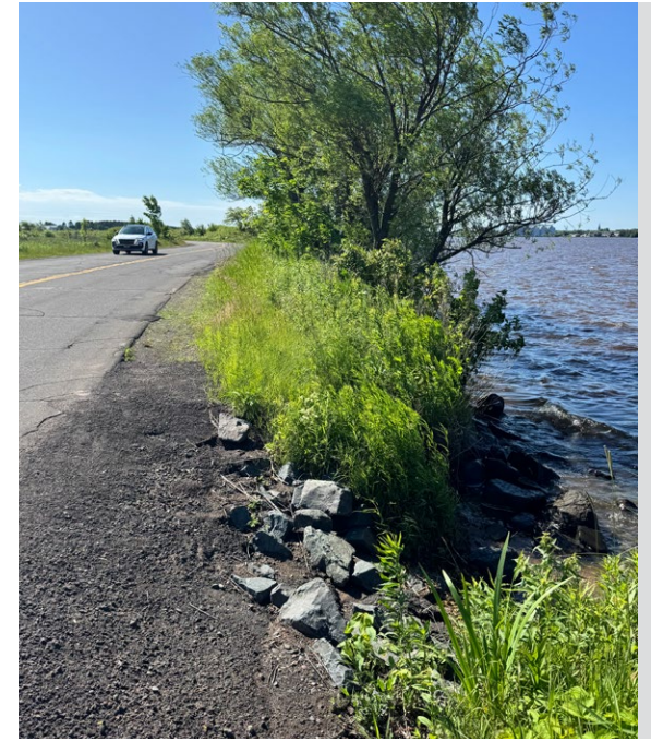
Figure 02.35 Existing narrow shoreline with erosion
