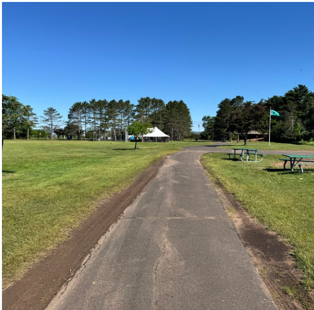
Figure 02.29 Erosion wear and tear along path (left)
