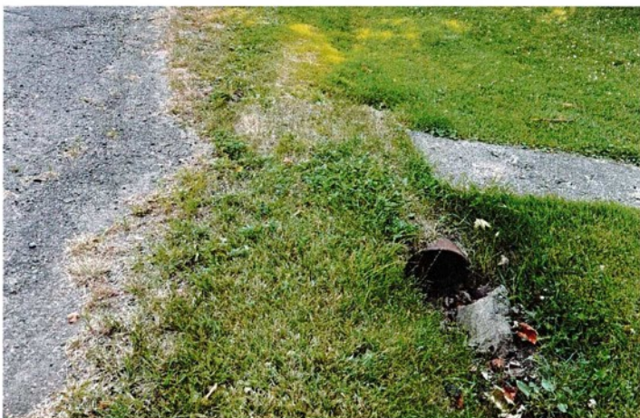
Pipe heave under catwalk on Springvale Road.
