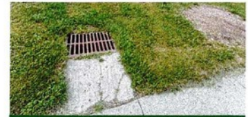
Existing catch basin condition on West House Street located outside of the flow line.
