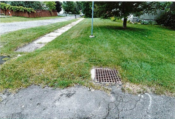
Existing catch basin condition on 98th Avenue West.
