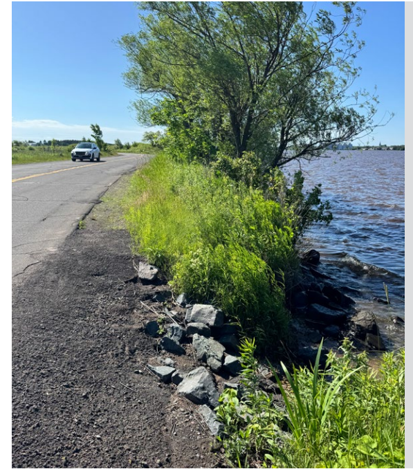
Figure 02.35 Existing narrow shoreline with erosion
