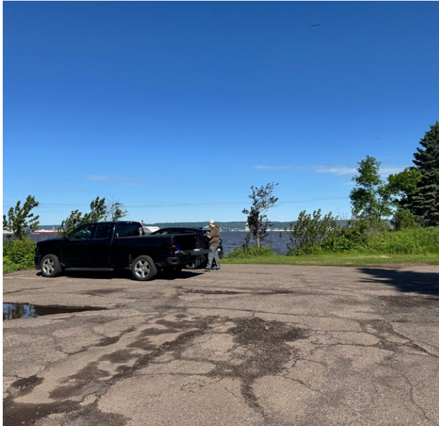
Figure 02.18 Trailer parking flooding (left)
